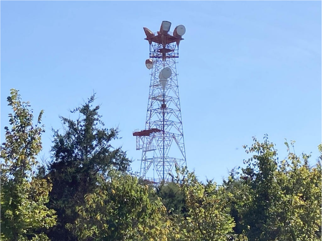
The antennas facing the camera from this angle are aimed toward Prairie Home. The opposing side is aimed toward Hermann.
